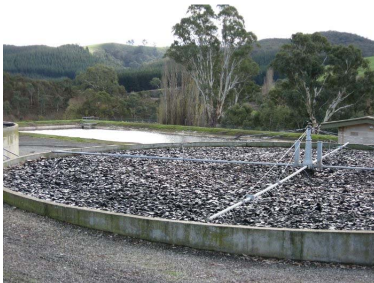
Figure 14.1 Gumeracha Wastewater Treatment Plant
