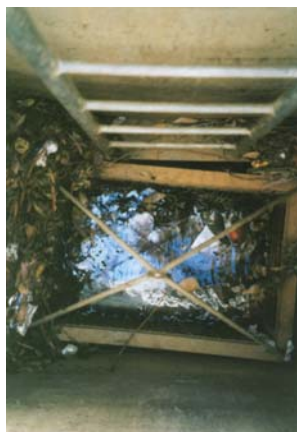
Figure 9.2 Inside a GPT
