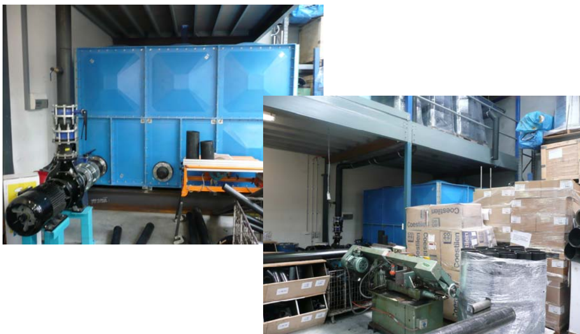
Figure 16.16: In-building Tank Fitted into the Space below a Mezzanine Walkway
