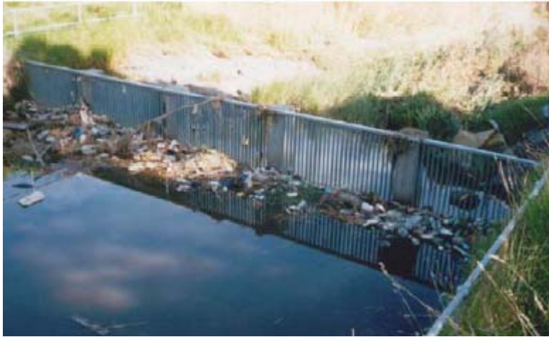
Figure 9.8 Trash Rack Installed at Broadmeadows, Victoria
